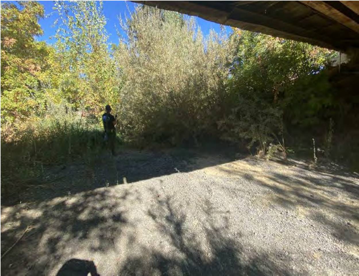
SITE 12- UNABLE TO REACH LOCATION, DENSE VEGETATION BLOCKING ACCESS
